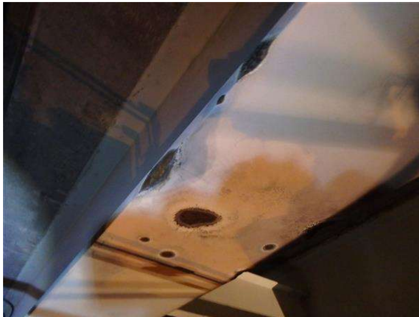
Typical melting section loss at girder G1 over track 1, typical.
