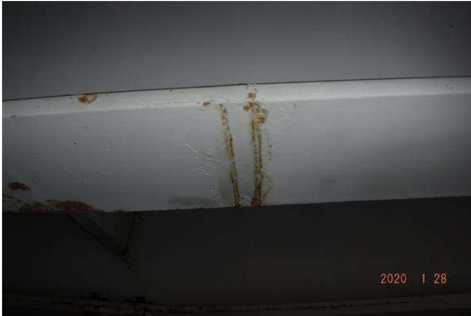
Span 8, Girder G6 bottom of bottom flange near Pier 7 has two (2) impact gouges.
