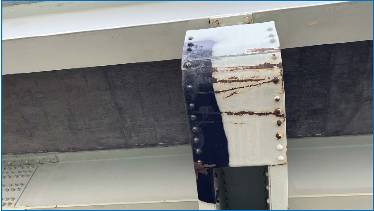
Photo 15: Minor Collision scrape at Pier Cap 3.
