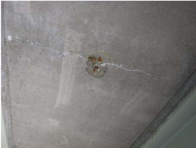
Span 6, Bay 3 underside of deck between Diaphragms D2 & D3 near Diaphragm D3 has a spall with an adjacent hollow area over the parking lot below.
