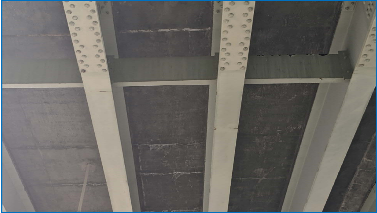
Photo 17: Underside of concrete deck. Random transverse cracks, active efflorescence, and isolated spalling. (Span 6 Girders 8 and 9 in photo).
