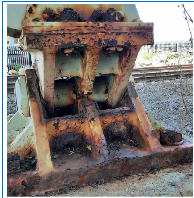
Photo 28: Pier bent bearing under pier 4 showing heavy laminar rust and pack rusting between plates.
