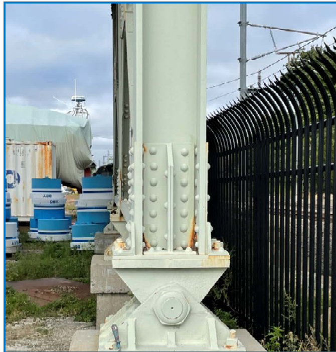
Photo 30: Elevation of Pier 3 column and bearing. Note laminated rust and section losses on interior column legs near bases.
