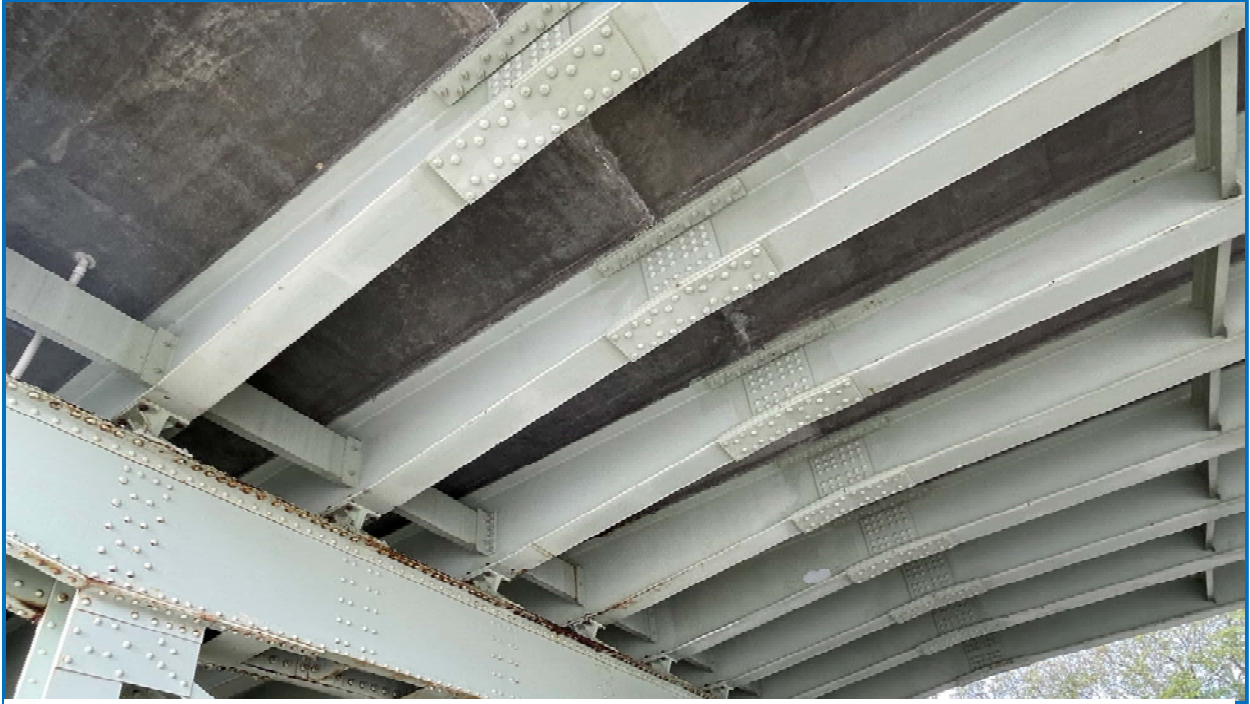
Photo 21: View under Span 8 showing flange transition and field splices adjacent to Pier 7.
