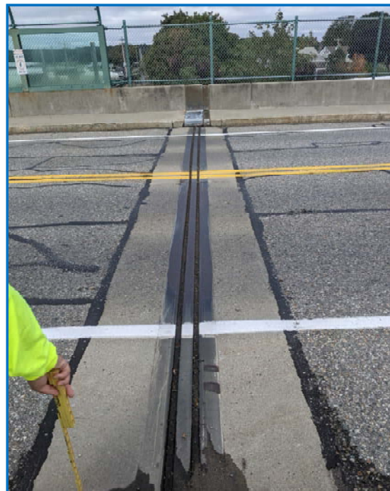
Photo 6: Condition of modular expansion joint with concrete headers over pier bend 4.
