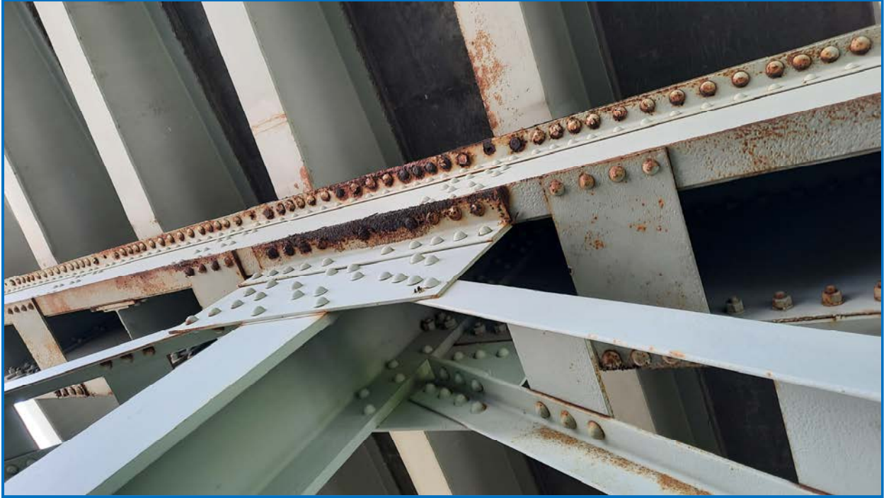
Photo 27: Pier Cap 6 top and bottom flange deterioration over center column. Photo taken from South side of pier.
