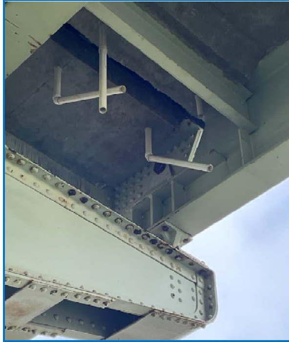
Photo 9: Bridge deck weephole drains extended to prevent drainage onto structure below (location in photo over pier bent 4).
