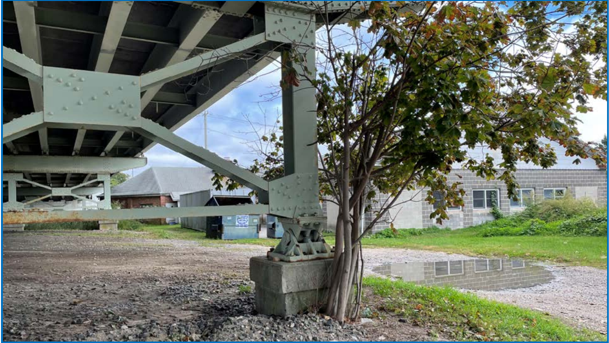
Photo 29: Tree growing beside bearing pedestal under Pier 5.
