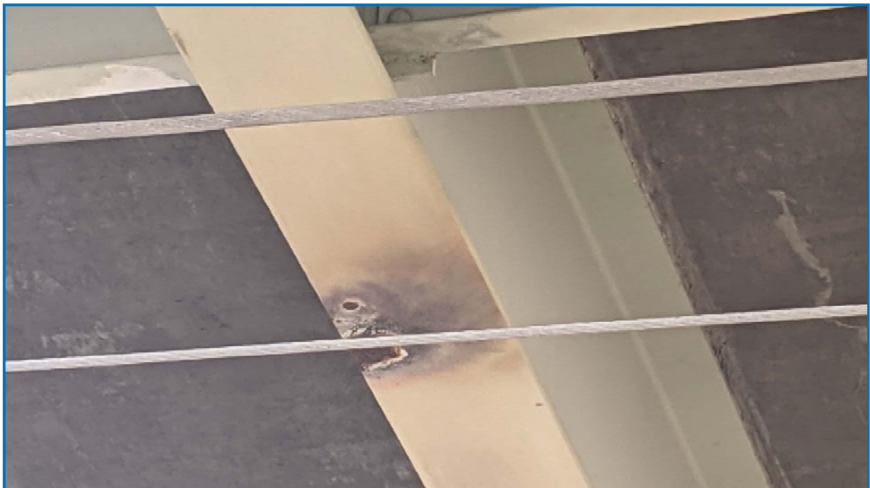
Photo 16: Typical Span 4 girder 2" diameter x 1/8" deep section loss due to electrical arcing over Amtrak rail lines.
