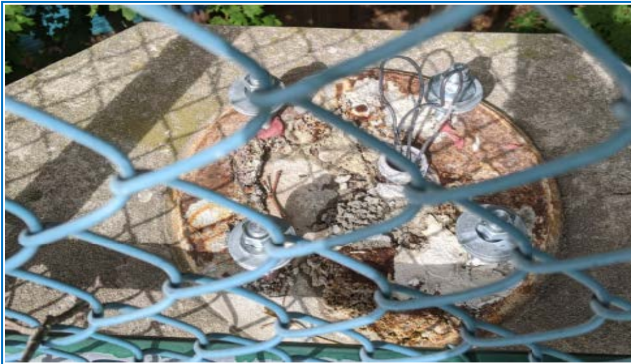
Photo 10: Close up of missing lighting standard at Span 3 west parapet.
