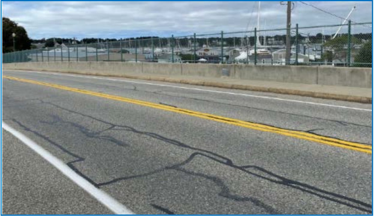
Photo 5: Condition of deck overlay showing transverse and longitudinal cracks (typical).
