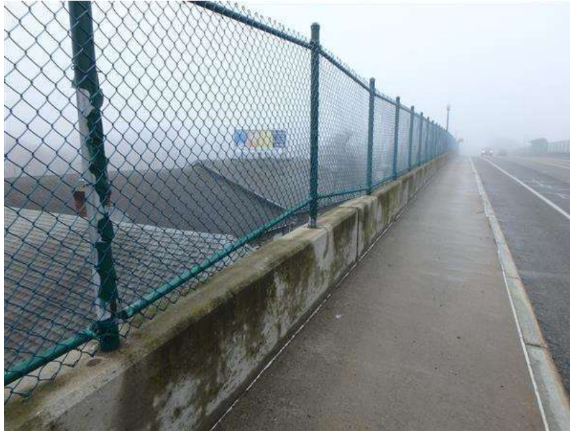
General view of the east sidewalk, parapet and fence. Note the fence post partially lifted out of parapet causing a gap between the fence and top of the parapet in span 7. Also see photo 13.
