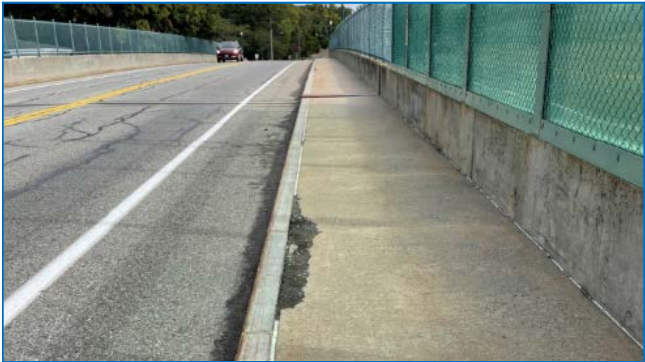
Photo 12: Sidewalk located on south side of bridge (looking North). Isolated areas on sealant and concrete missing behind the granite curbing (typical).
