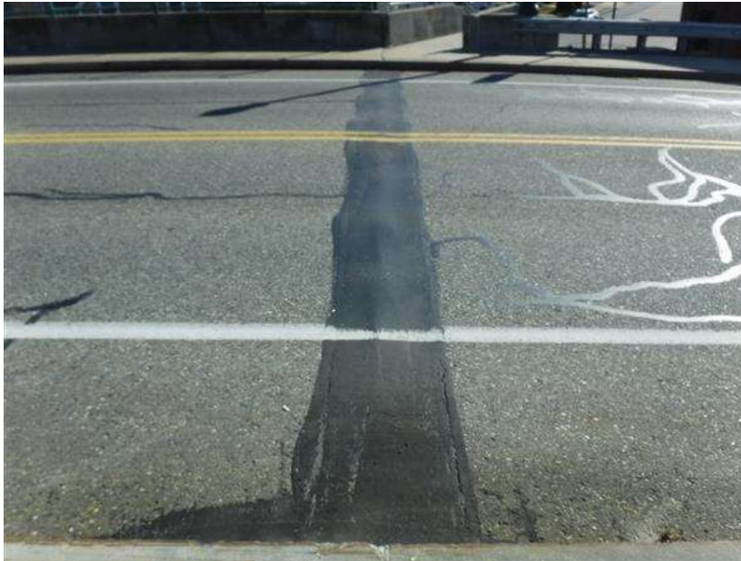
Abutment 1 plug joint has multiple adhesion cracks with full length settlement/depressions, looking east.
