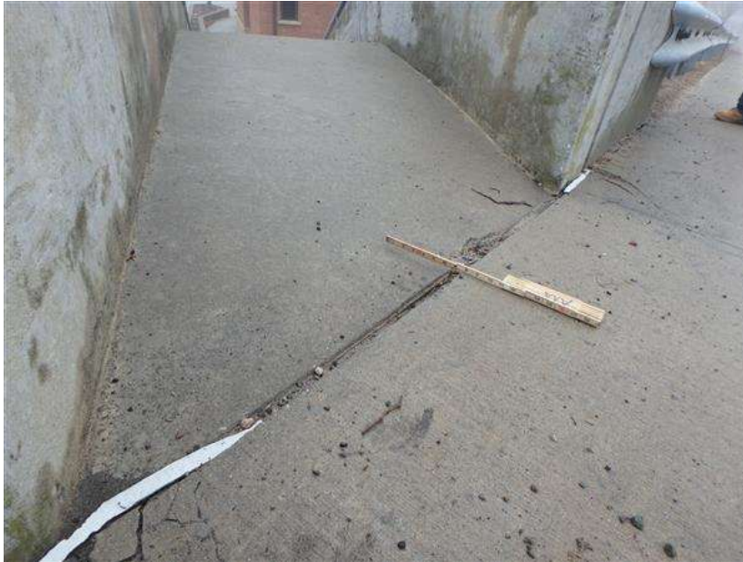
Deteriorated sealant and vertical misalignment at the southeast staircase and southeast approach sidewalk.
