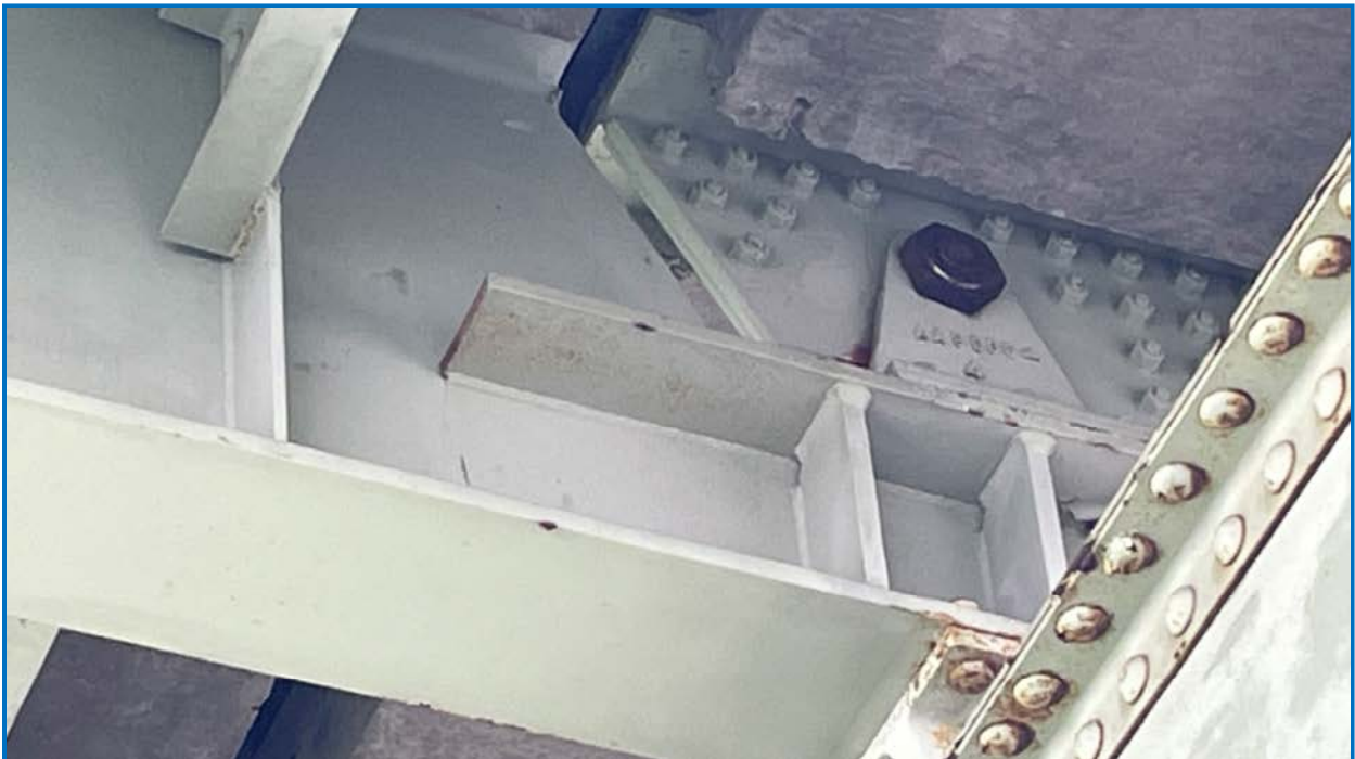
Photo 14: Expansion bearings over pier bent 4. No paint over the nuts or bearing pins (typical).
