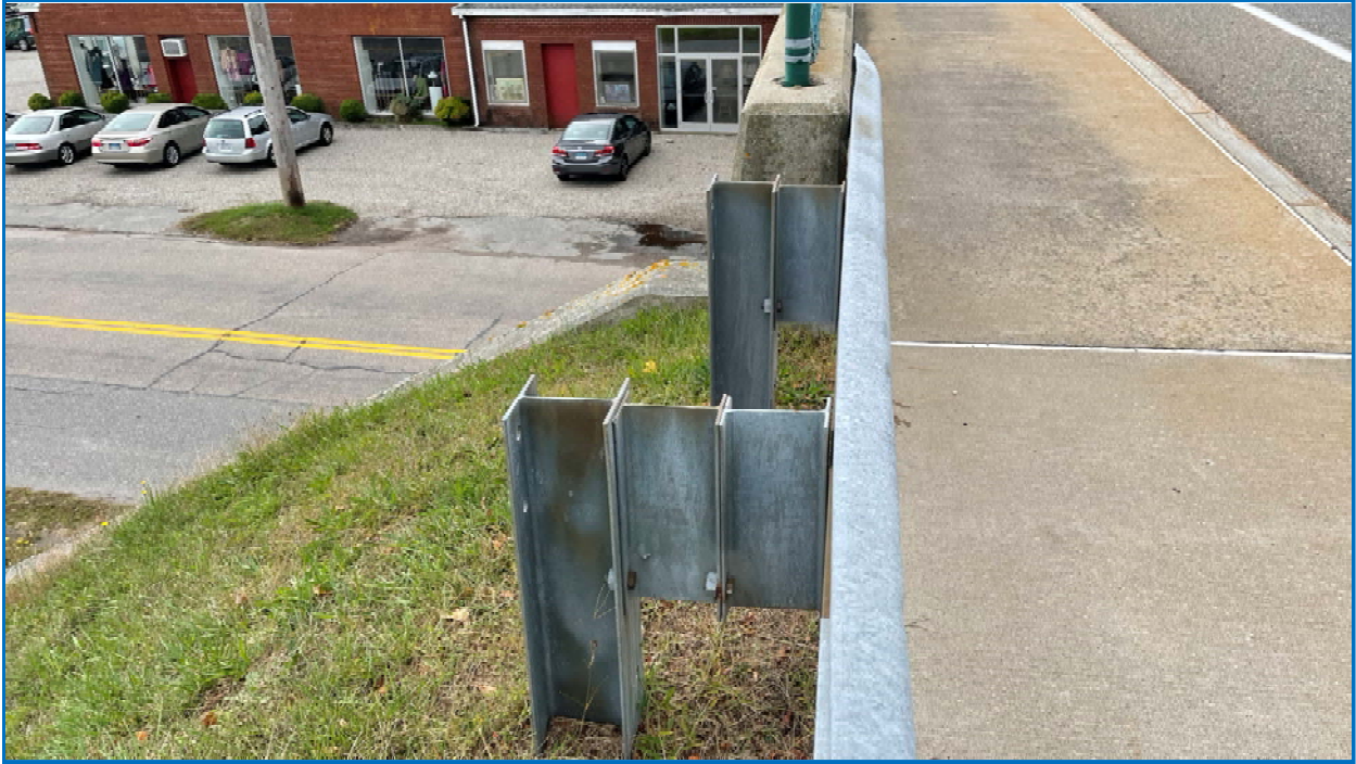
Photo 33: Metal Beam rail with steel posts and block outs. Typical for all approach corners.
