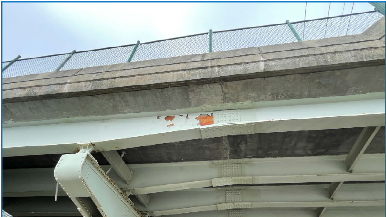
Photo 22: Facia of Girder G9 in Span 8 showing areas of peeling paint and surface rust near field splice.
