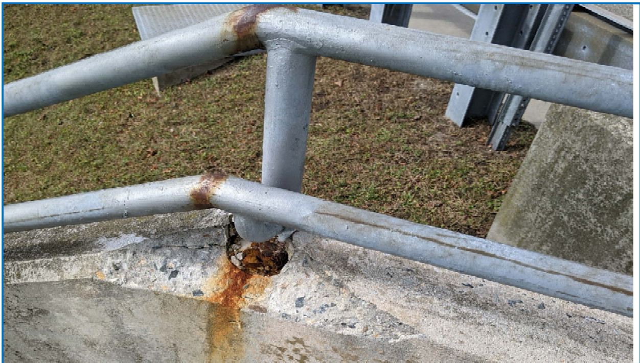
Photo 8: Condition of southeast stairwell showing spalled concrete and missing hand rail post.
