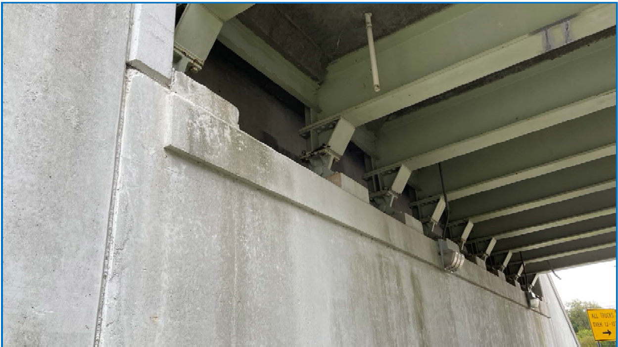
Photo 20: Abutment 2 adjacent to Cutler Street. Note scrape marks on bottom flange of Girder G2 painted over in top right of photo.
