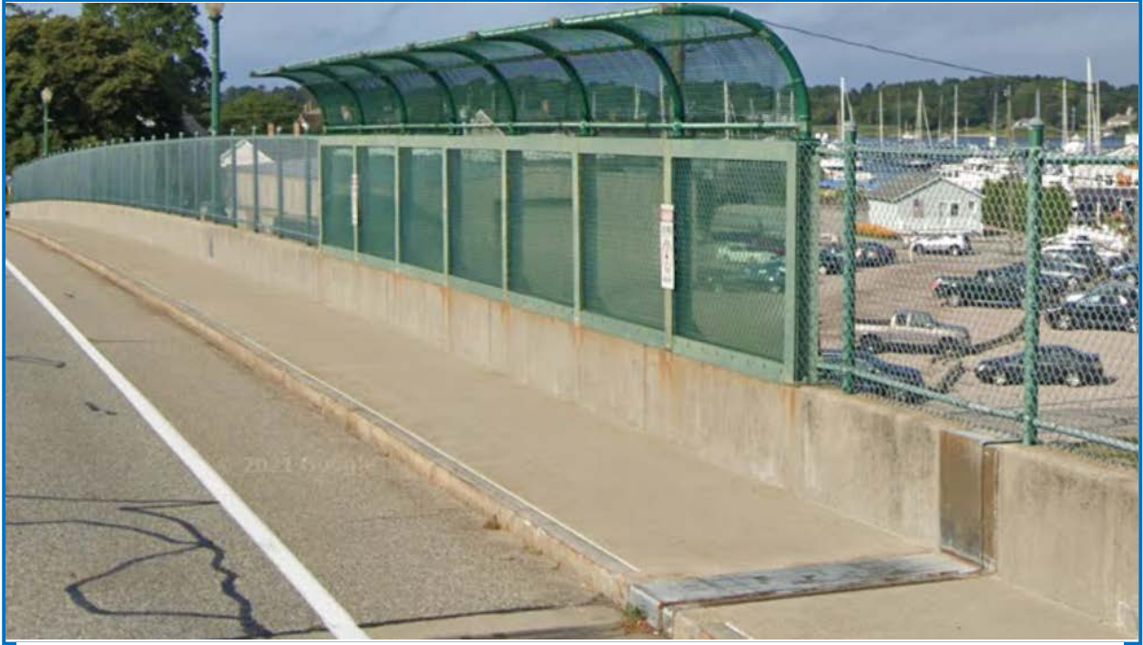
Photo 11: Condition of bridge parapets and vinyl coated chain link fencing.
