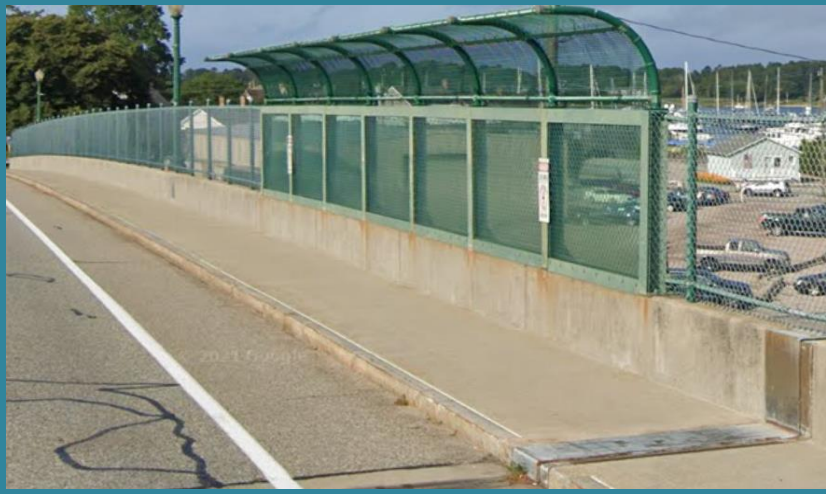
Condition of bridge parapets and sidewalks.
