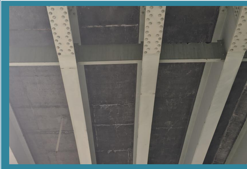
Condition of concrete deck showing random transverse cracks, efflorescence and isolated spalling (Span 6 shown).
