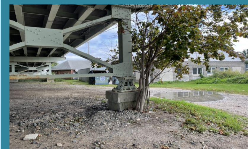
Tree growing beside bearing pedestal under Pier Bent 5.
