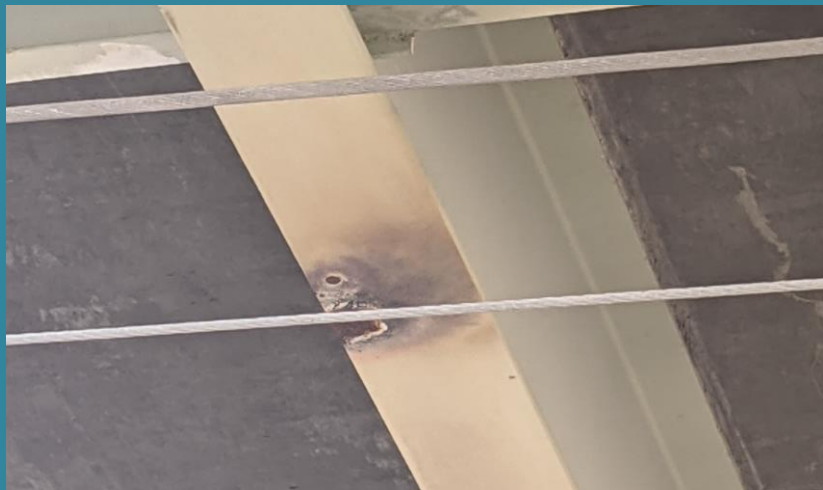
Electrical arcing over Amtrak Rail lines. Typical condition for Span 4 Girders.
