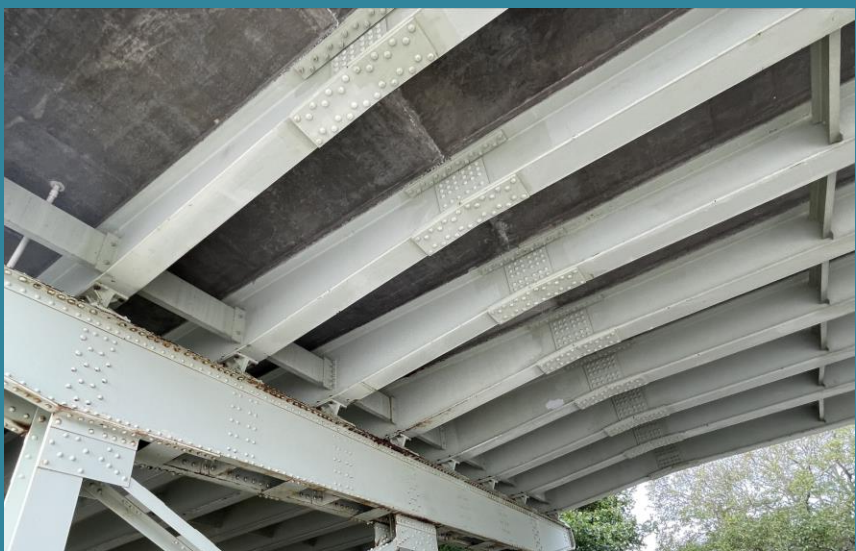
View under Span 8 showing flange transition and field splices adjacent to Pier Bent 7.
